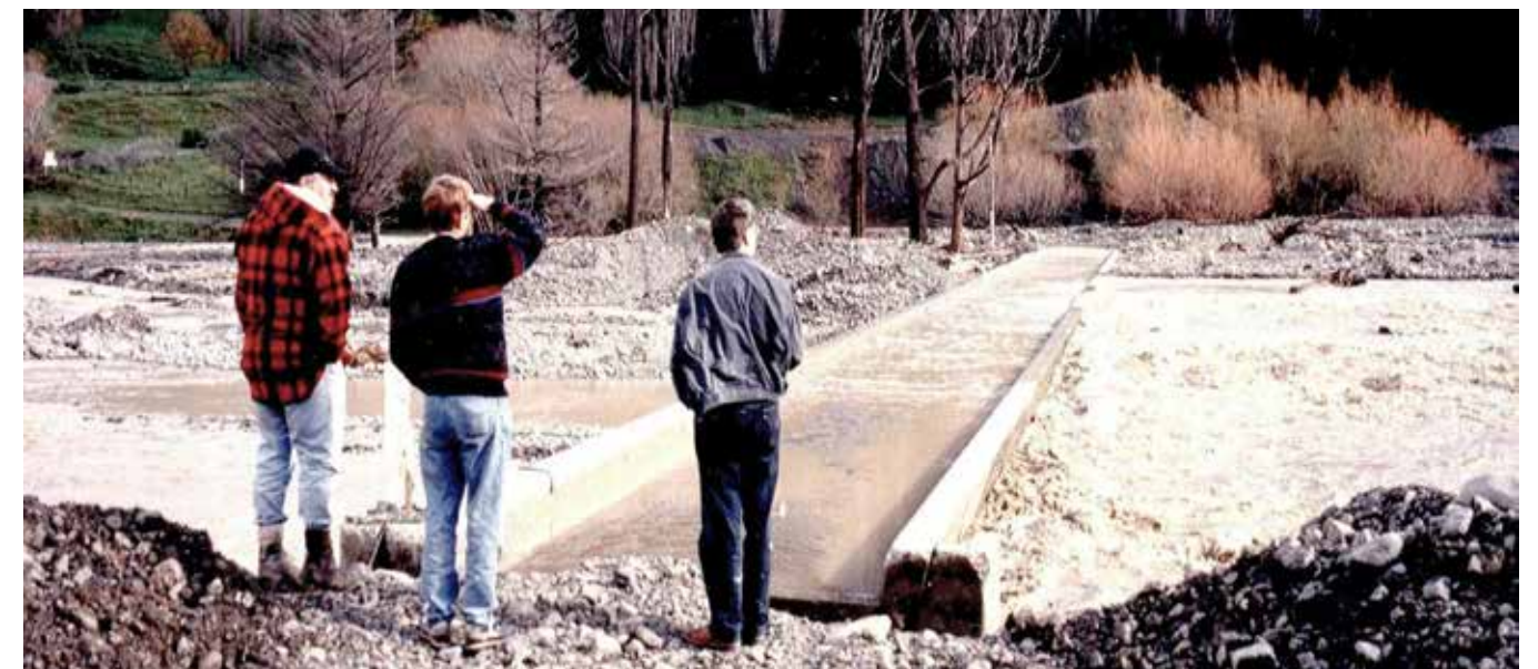
Aggraded riverbed after Cyclone Bola – the bridge (over the Raparapaririki River inland of Ruatorēa) is now buried under several metres of gravel
